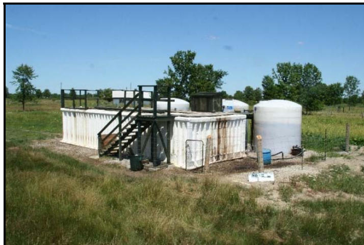
Figure B-27: Feature NB-N, brine separating system. Since the 1980s, the brine must be separated from the oil and injected back into the ground
