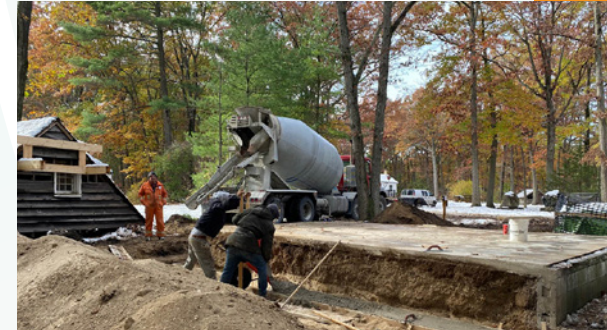
Concrete footings are poured as part of the foundation for the reconstruction of the historic Canatara Cabin at LHM.
