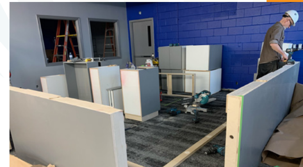
A new accessible service desk is installed as part of the renovations to the former community hall at the Clearwater Arena in Sarnia, in preparation for the opening of the new Clearwater Library, scheduled for February of 2024.
