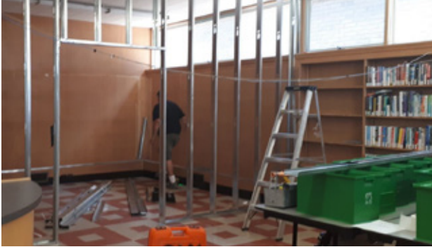
Contractors build a new private meeting space as part of the Social Services Integration project at Corunna Library.
