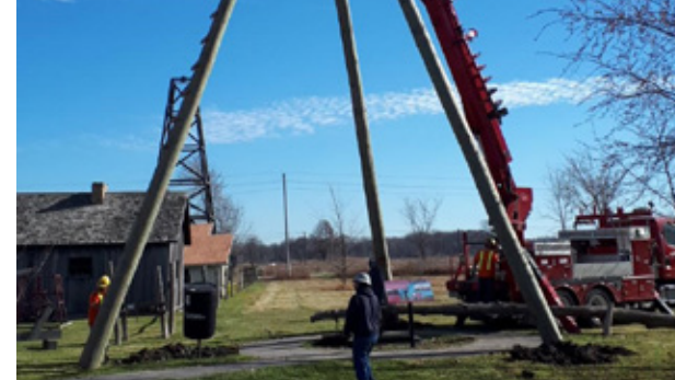
OMC staff work with Bluewater Power and community volunteers to install a replacement three-pole derrick on the museum property.
