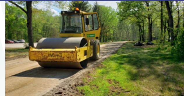
The main driveway at LHM is prepared for new asphalt, as part of parking lot and accessibility improvements at the museum site.
